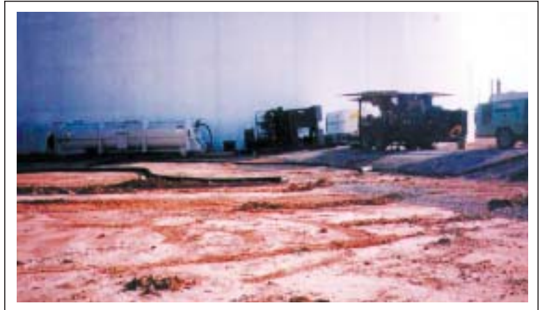
All UHP equipment is located outside the tank
