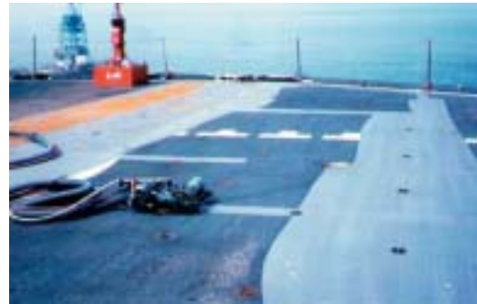
Clean steel is left with its existing profile intact ready for recoating
